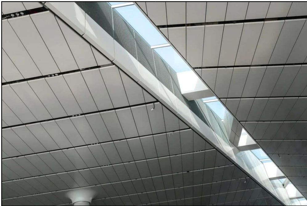
Figure 2-20: Lighting and conditioning systems. (Source: architectural review: Online)
