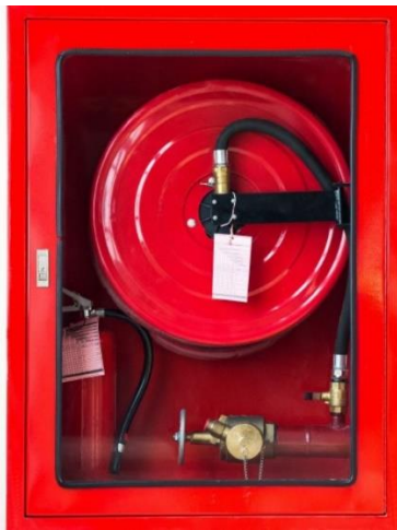
Figure 203 Hose terminal station
