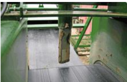
Figure 12:Hydro-Probe installed above sand conveyor belt
