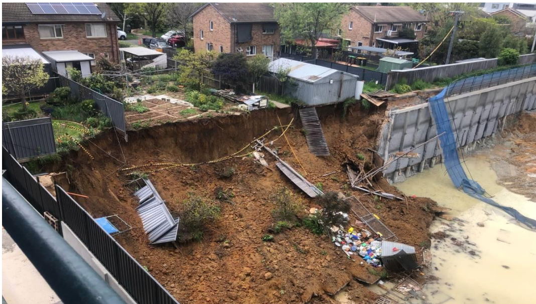
Figure 3.2: Shows a Case of Retaining Wall Getting Collapsed at a Construction Site
