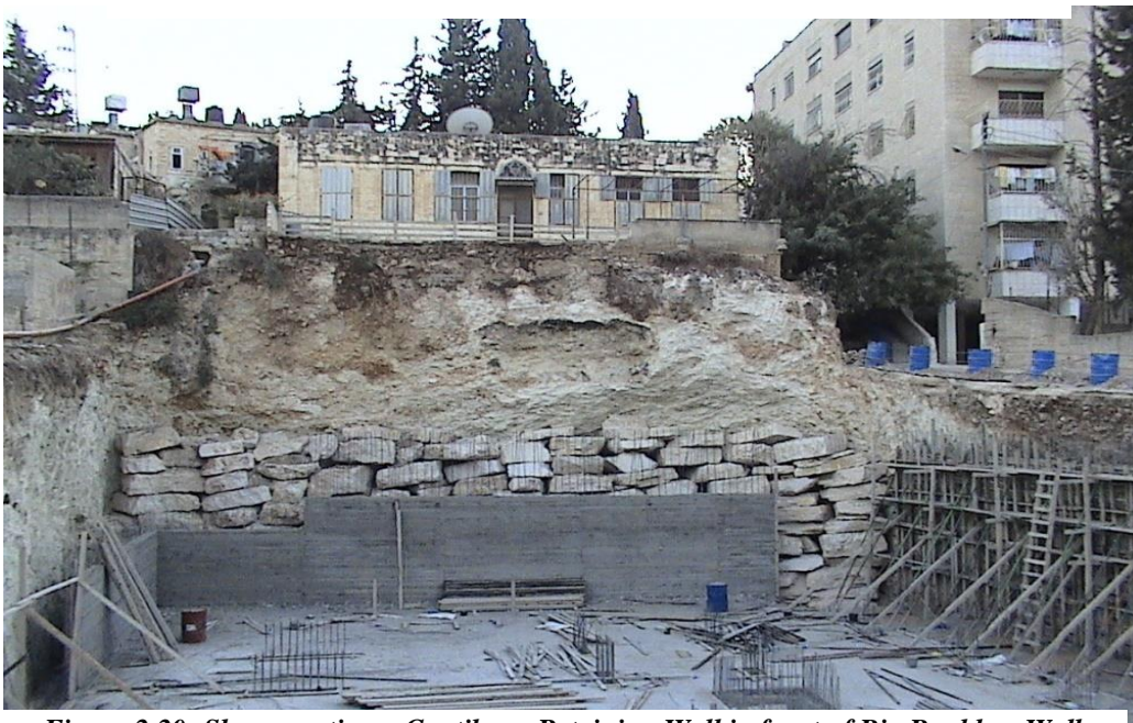
Figure 2.20: Shows casting a Cantilever Retaining Wall in front of Big Boulders Wall
