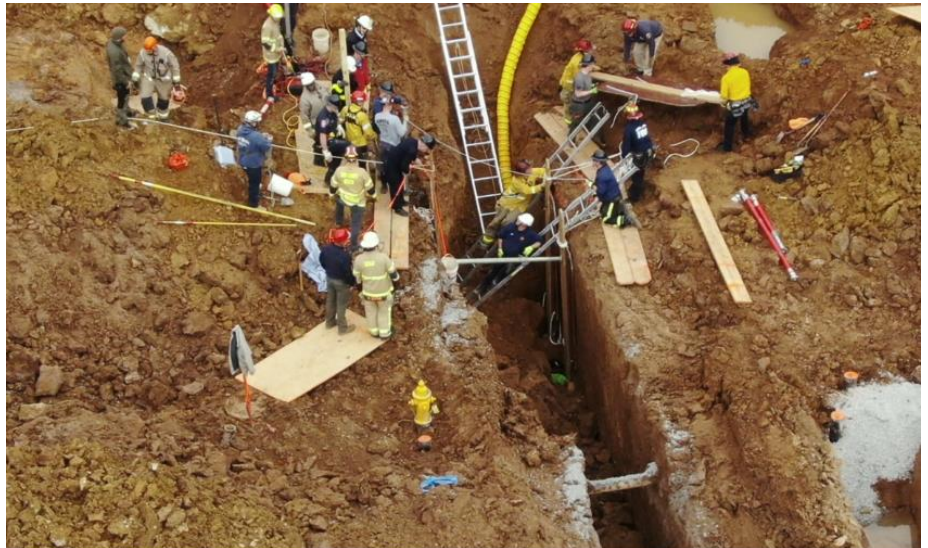
Figure 3.1: Shows a Trench Collapse and two workers are being rescued near Knoxville
