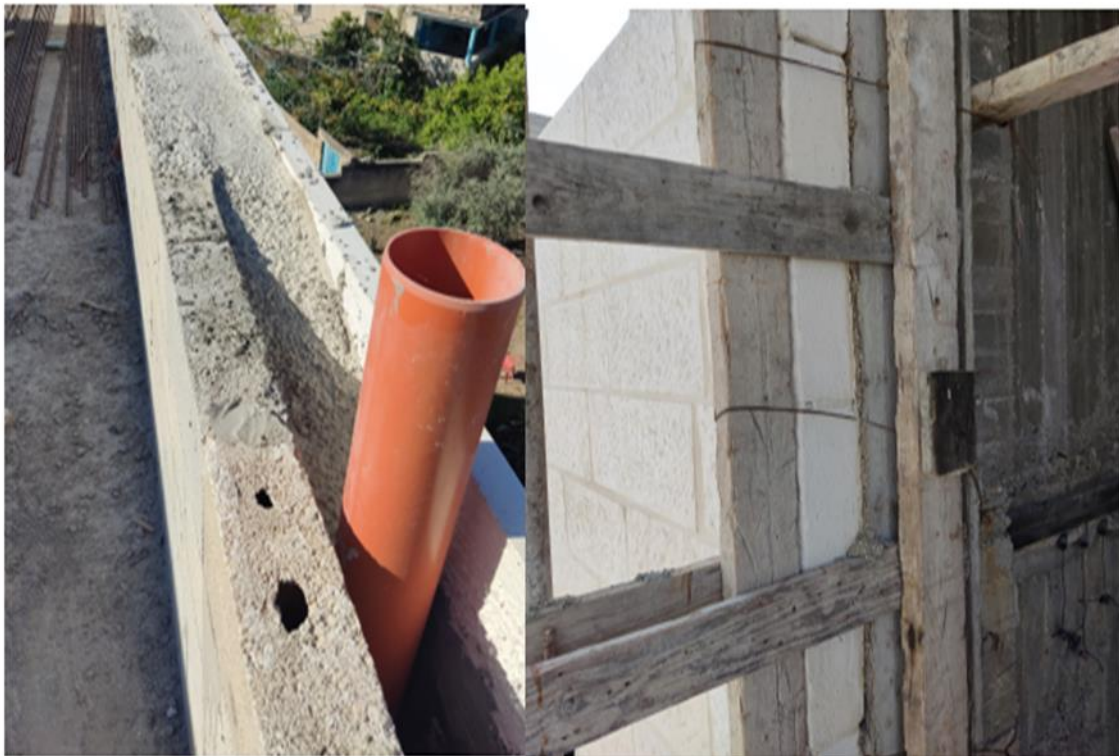
a) Using 10 cm hollow brick as a permanent shutter b) Using wood shutter
