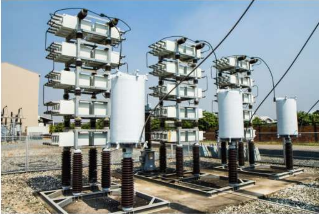
Figure 5: Capacitor bank for substation.
