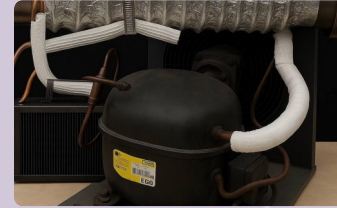
Copper pipes with circulating refrigerant (compressor + radiator).
