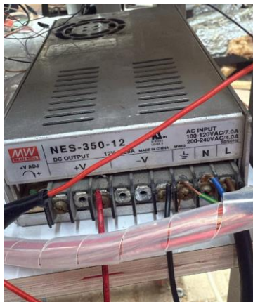
Figure 3 Switching Power Supply
