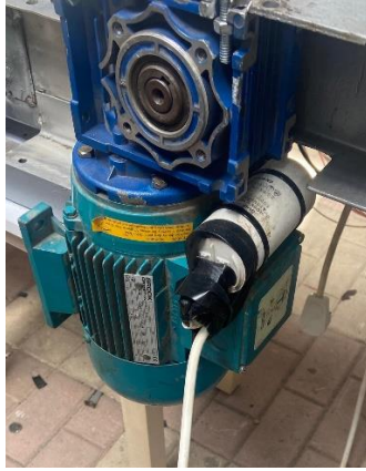
Figure 16 Chinese water pump motor
