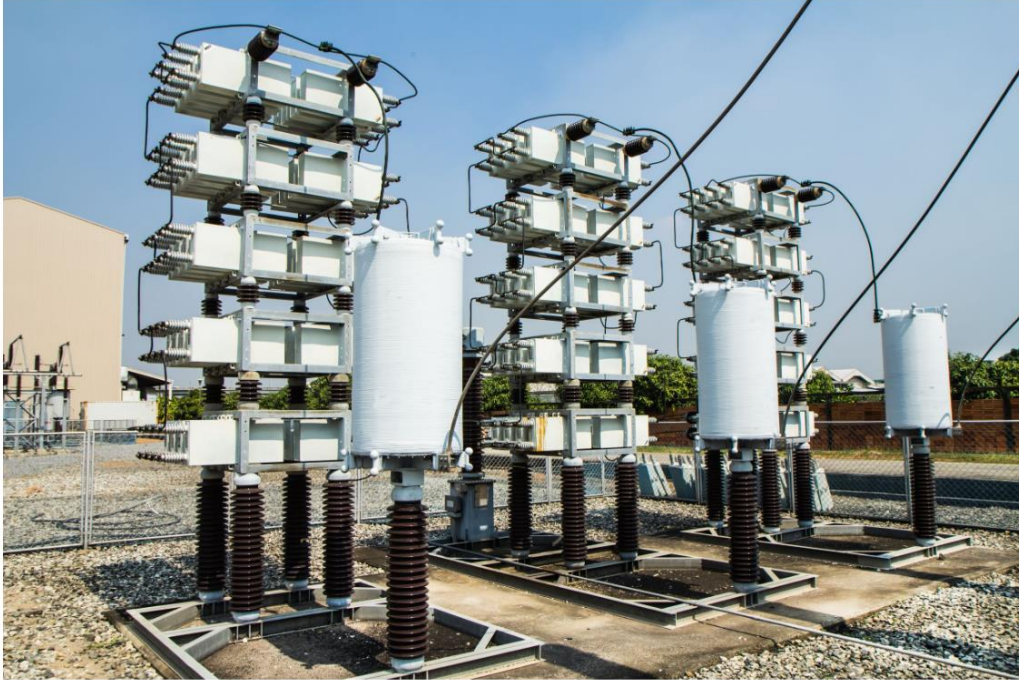
Figure 5: Capacitor bank for substation.
