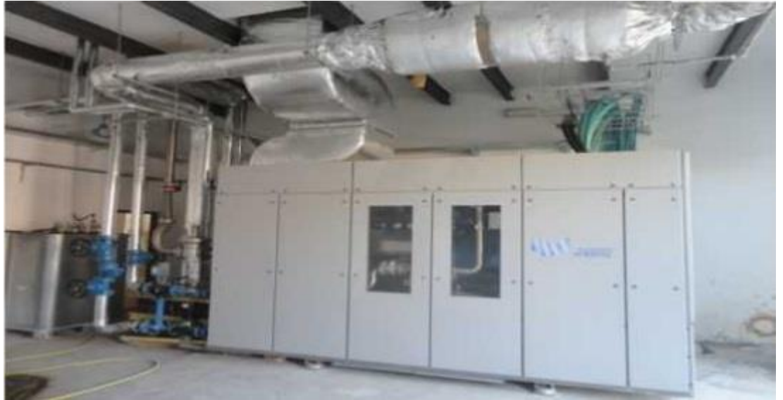
Figure 2.13: Recently Operated CHP unit
