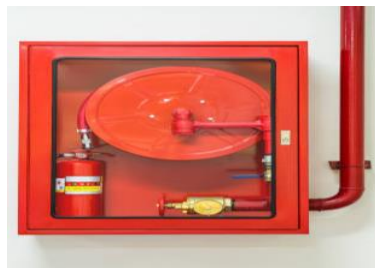
Figure 169 fire hose station
