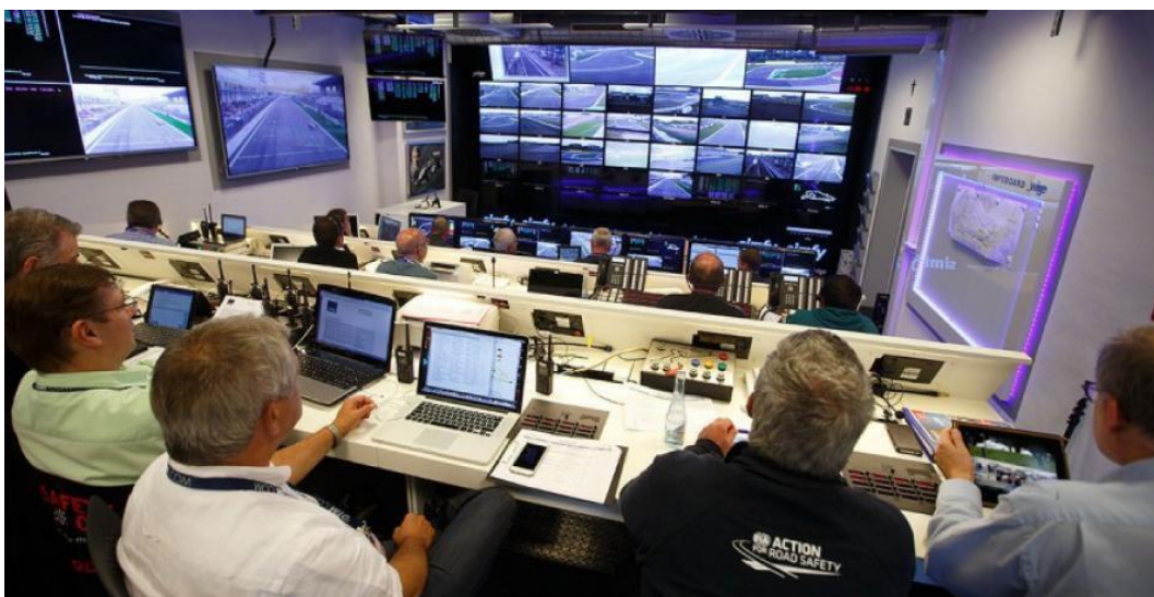
Figure 4.43: Control Room Interior
