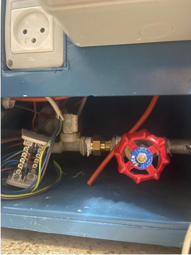
Figure 3.14: Manual valve & Electrical valve.
