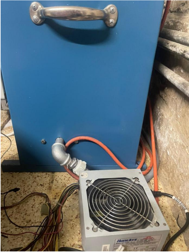
Figure 3.15: Power supply and main water source.
