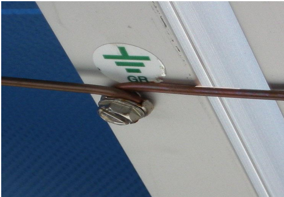
Figure (5.17): Improper Grounding PV module
