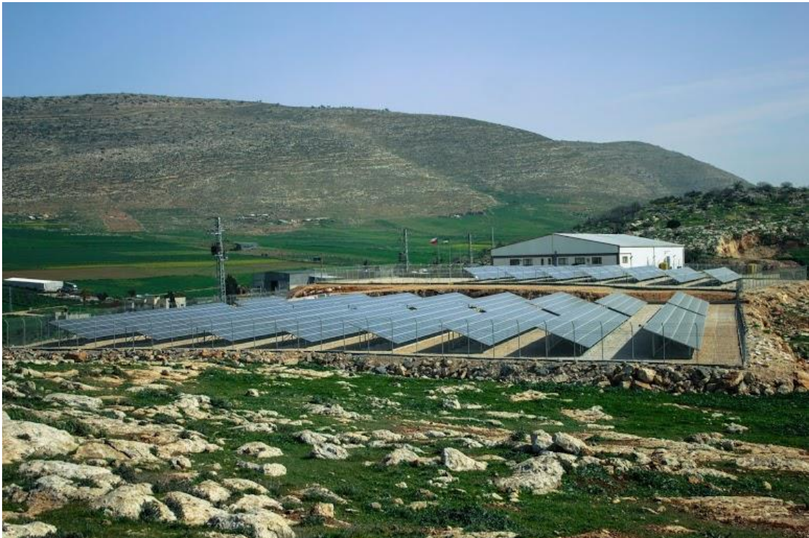
Figure (1.3): 470kWp TDECOs' PV Power Station
