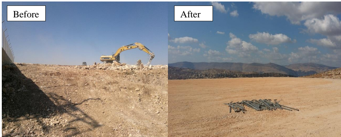
Figure (5.1): The Location of PV Power Station Before and After Land Preparation
