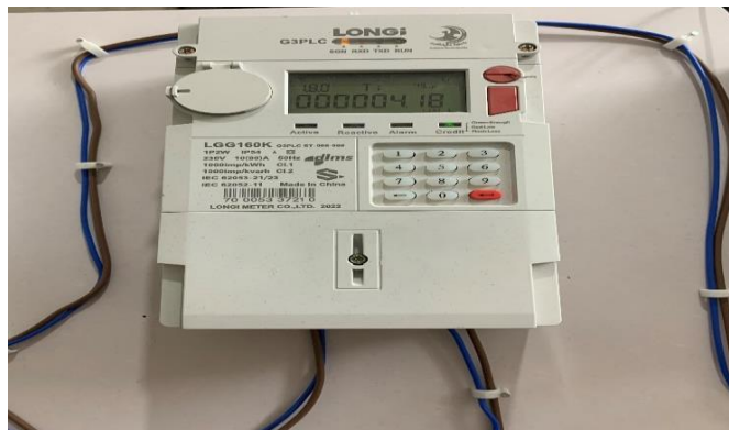
Figure 15: single phase smart meter.
