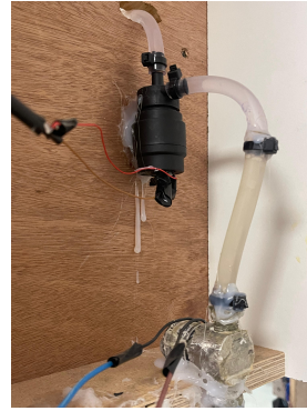
Figure 3.3: pump and valve
