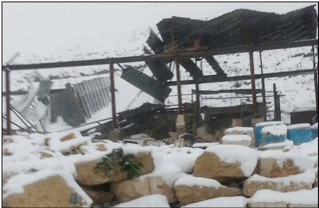
Figure B.14 Snow fall adverse effect on Jamaeen company truss
