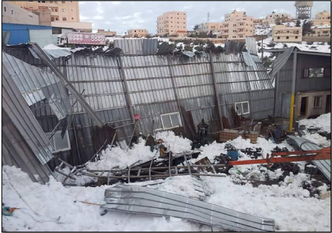
Figure B.4 Snow fall adverse effect on Shahatet company truss
