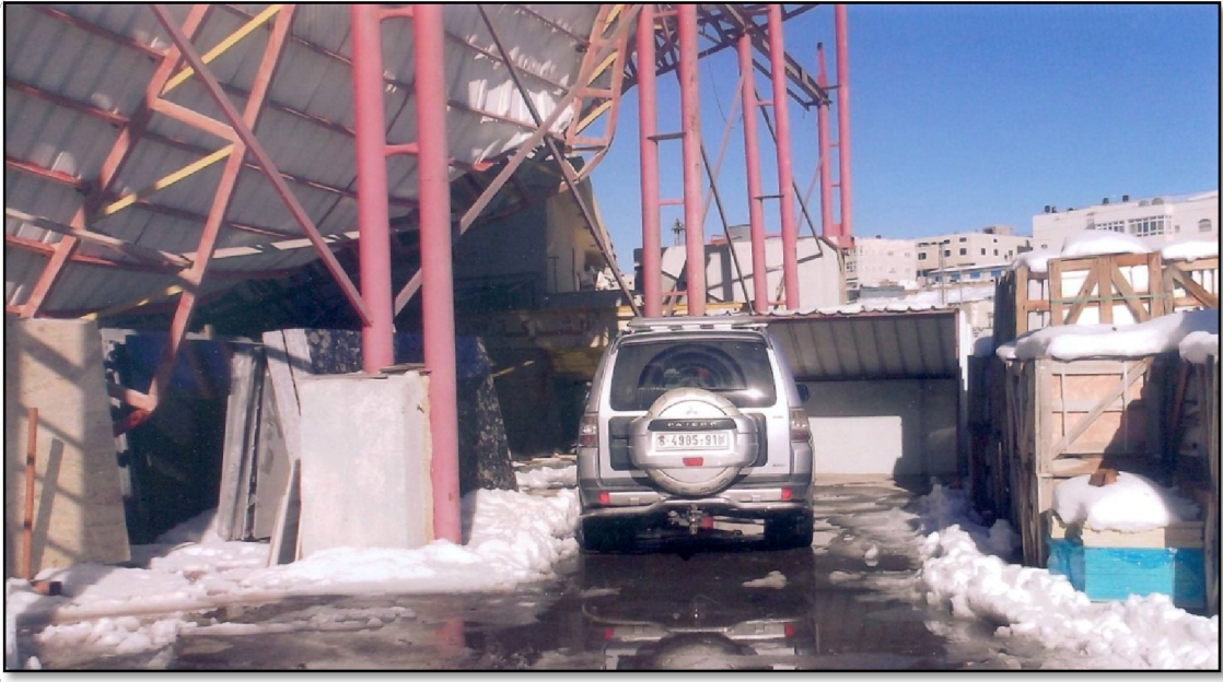
Figure B.9 Snow fall adverse effect on the Italian company truss
