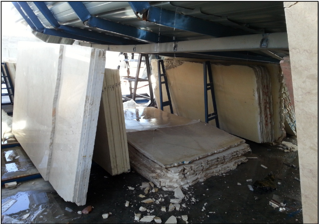
Figure B.12 Snow fall adverse effect on Geneva company truss
