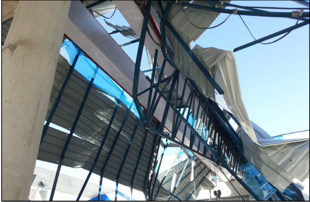
Figure B.13 Snow fall adverse effect on Geneva company truss
