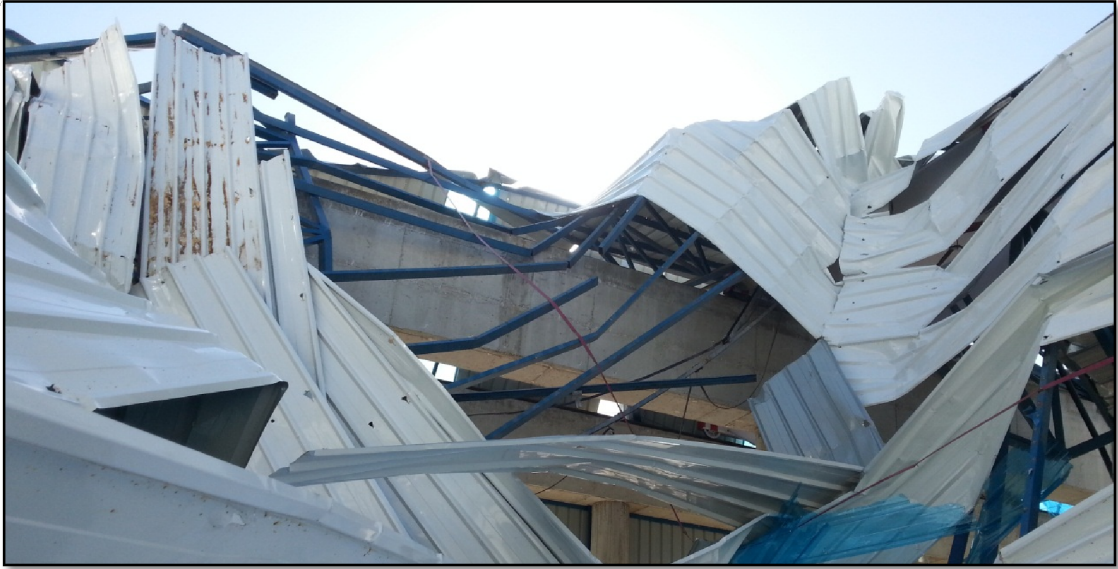
Figure B.11 Snow fall adverse effect on Geneva company truss
