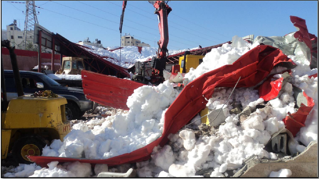
Figure B.7 Snow fall adverse effect on Al Mahabba company truss
