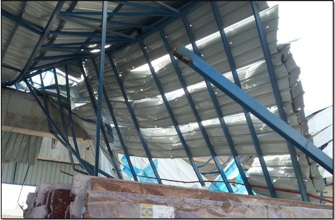
Figure (4.2): Snow fall effects on Geneva company truss.
