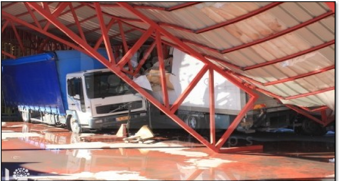
Figure B.6 Snow fall adverse effect on Al Mahabba company truss
