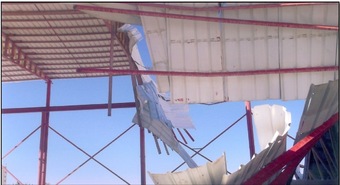
Figure B.8 Snow fall adverse effect on the Italian company truss
