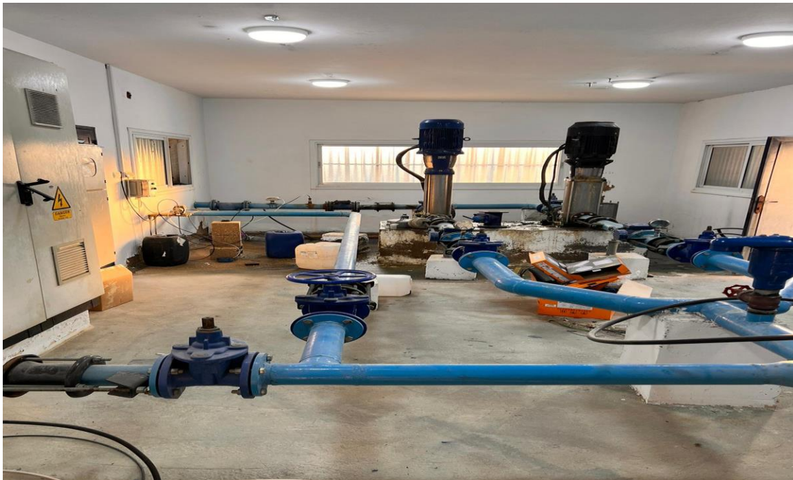
Figure 14 Yasid booster station
