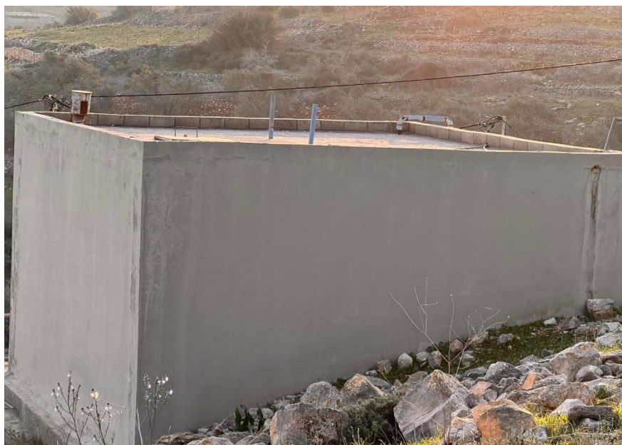
Figure 10 Storage tank I
