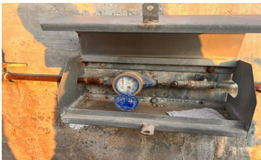
Figure 16 Mechanical water meter
