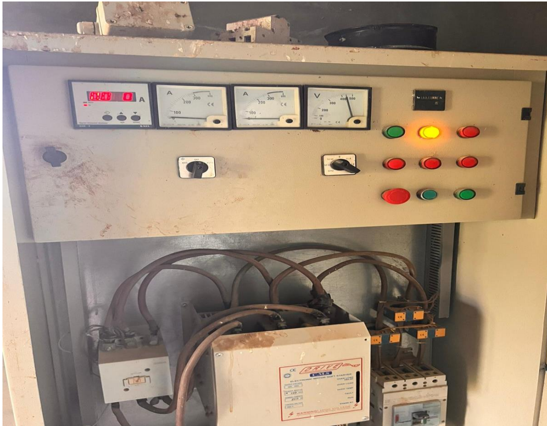
Figure 15 Controlling device for Yasid Pump and booster's station
