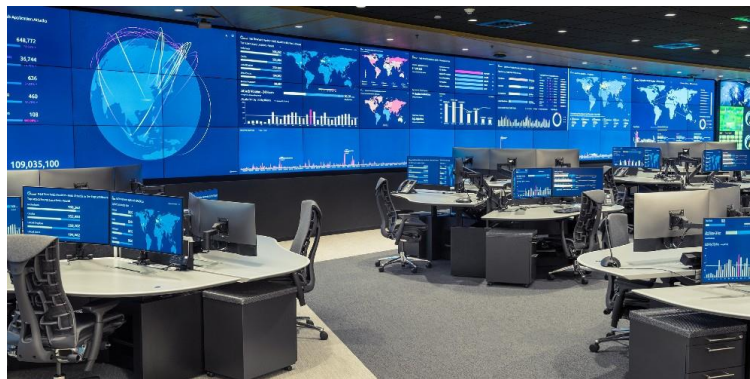
Figure 3 Network Operations Center
