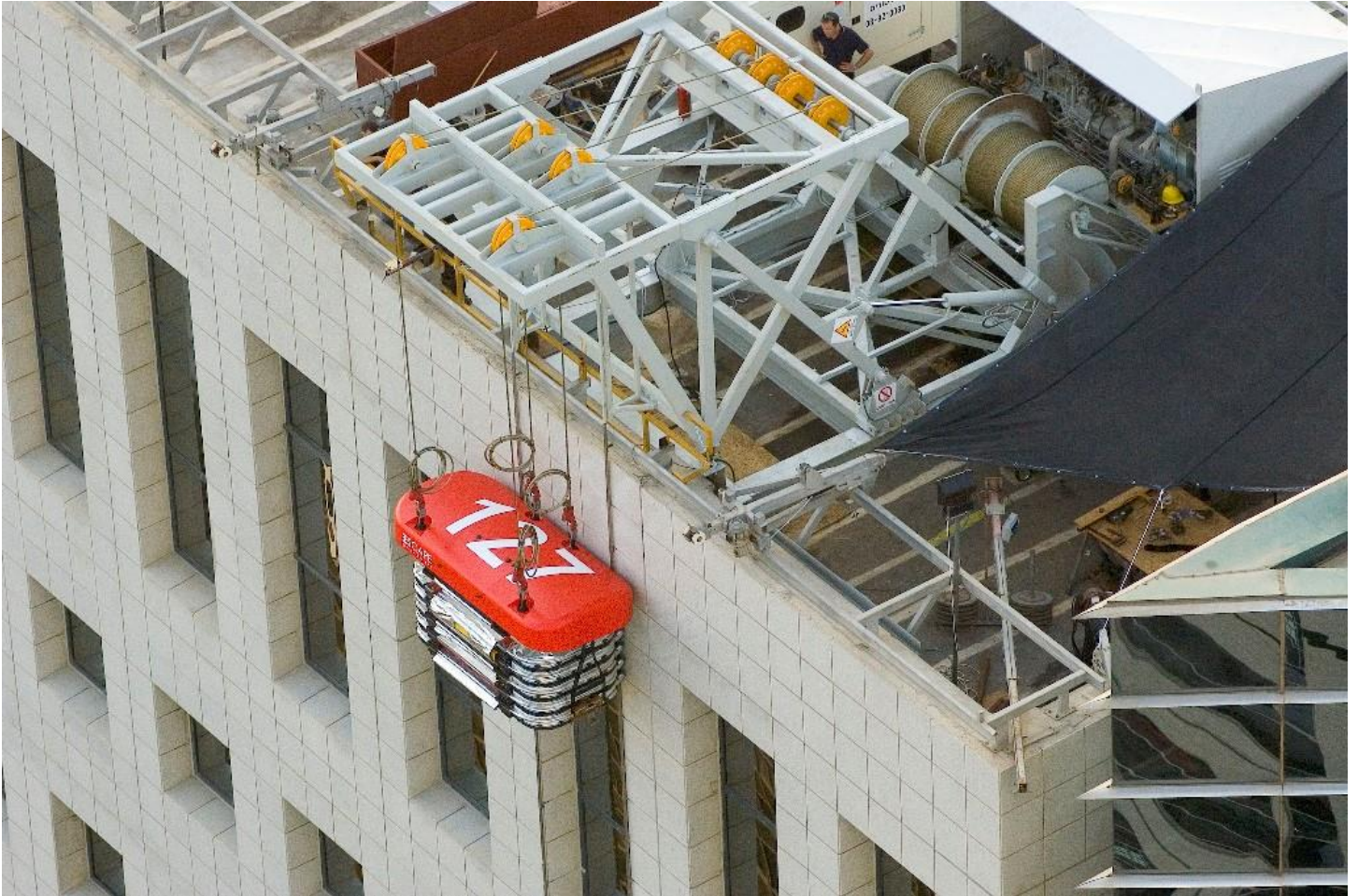
Figure 310 emergency elevator (escape and rescue system, n.d.)
