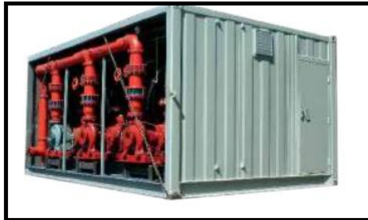
Figure 260: Fire pump used. (Fire Extinguishers, 2021)
