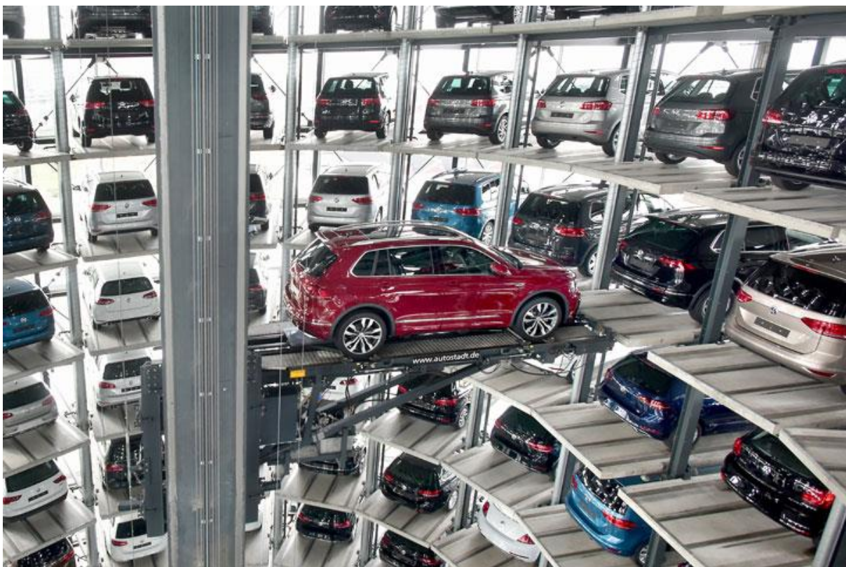
Figure 5.d: Automated (Robotic) Parking System
