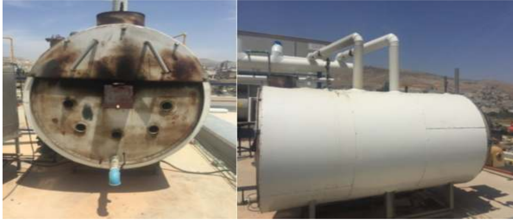
Figure(25):Al-Arz factory LPG boiler (Al Assi and Tayeh, 2016).
