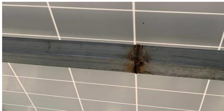
Figure 8: Welding support problem
