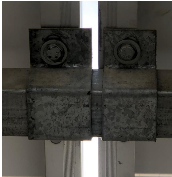
Figure 6: Chassis-modules support problem1
